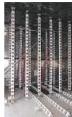
The HD 200 props are used for their high load capacity in this relatively confined workspace. Loads were transferred from the slab to the steel beams and then to the HD 200.
