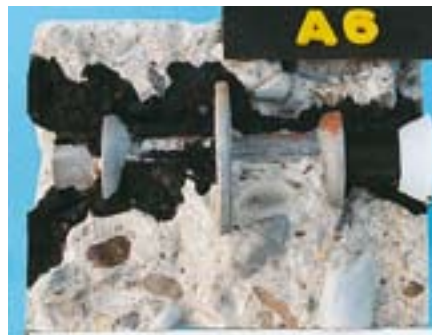
...and cast-in waterstop centrepieces likely to leak.
